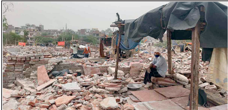
Residents of Bengali Camp in Chhuriya Mohalla of Delhi's Tughlaqabad village sift through the rubble of their homes after they were demolished in April 2023. Credit: Sneha
